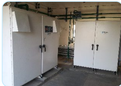
20 Nm 3 /hr Hydrogen Generator at Power Plant in M.P.
