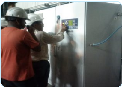
6 Nm 3 /hr Hydrogen Generator Installed inside TG Building in U.P.
